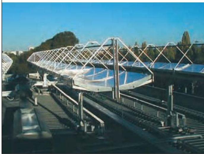
Concentratore CHAPS (Combined Heat and Power Solar) (ANU) AUS
